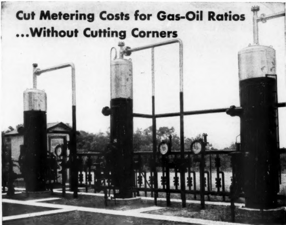
Measuring gas from Separator Batteries at Conoco Driscoll Field, Benavides, Texas with 3 Foxboro Gas Flow Meters Type 4.
